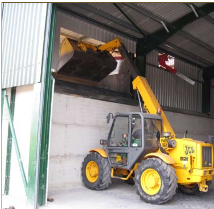
This roller shutter door, inside the building, provides access to the 20ft capacity intake hopper. Rubber matting on the loading lip helps contain any spillages.
